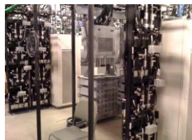
Wireless Carrier Facilities
